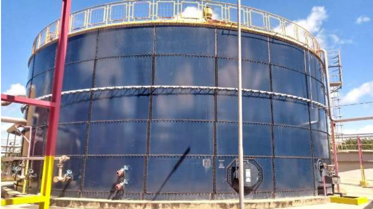
Figura 21 – UASB ( Upflow Anaerobic Sludge Blanket ).
