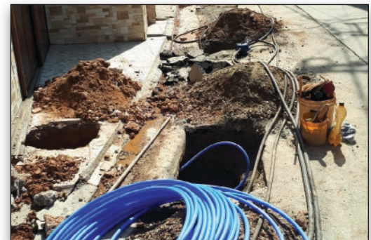
All updates implemented during the first phase of construction improved the water supply to the residents of Diadema.
